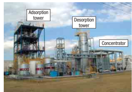
Solvent recovery facility
