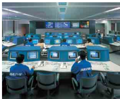
Control center monitors and controls buildings 24 hours a day and responds to emergency calls.
