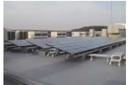
Solar power system introduced at Hitachi System Plaza Okayama
