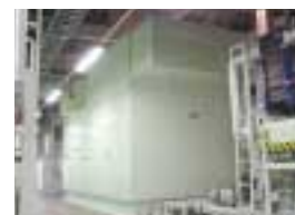
Sapporo Breweries, Ltd. Hokkaido Plant, gas co-generation facility
