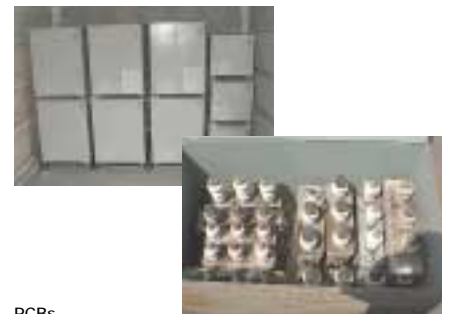
PCBs (An example of high-pressure condenser storage management)
