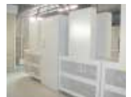
Sapporo Breweries, Ltd. Sendai Plant, refrigeration inverter facility
