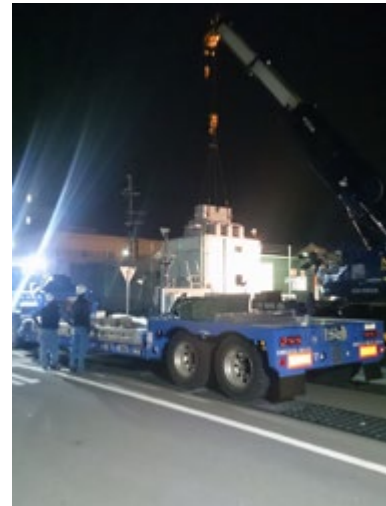
Disposing of waste materials (large transformers) containing PCBs.
