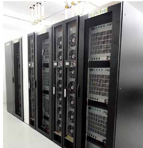
Modular data center
