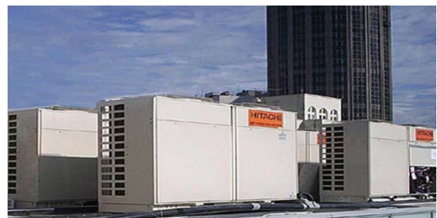
Fig. 6—Outdoor Units of Multi-split System Installed on Roof. The multi-split system is mainly used for office and apartment buildings. Because it can be installed on the roof, building space can be used effectively.
