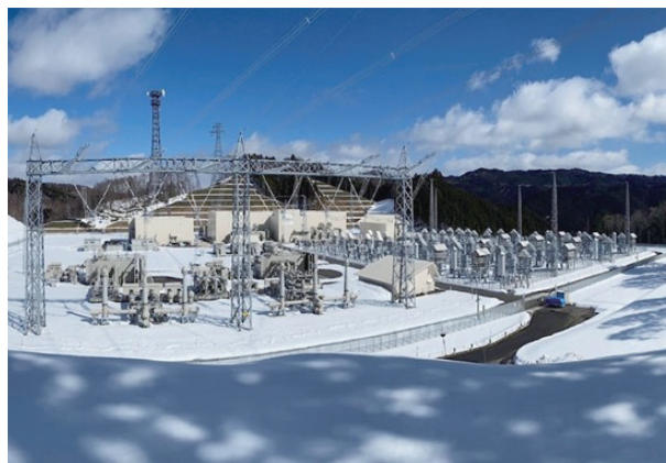
Chubu Electric Power Grid Hida Shinano Frequency Conversion Facility: Hitachi delivered a high-voltage direct current (HVDC) system to this facility. Hitachi Energy products are used in the AC filters.
