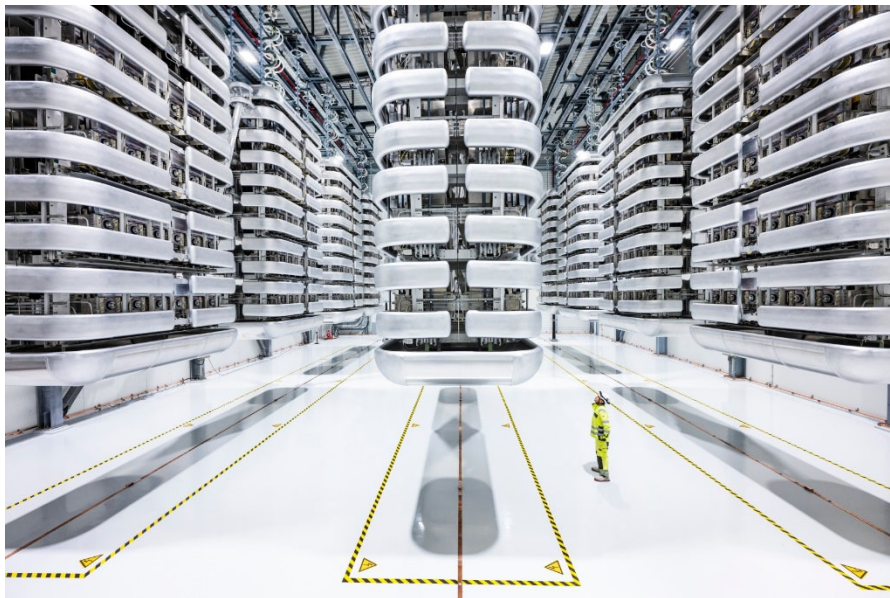
Hitachi Energy HVDC valve hall
