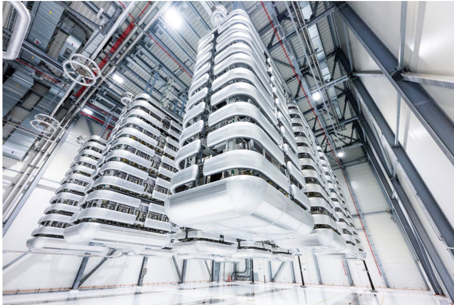
HVDC Light® Valve Hall
