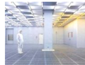
Clean room facility
