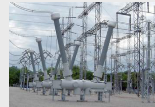
Gas circuit breaker
