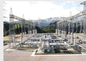
GIS: Gas Insulated Switchgear
