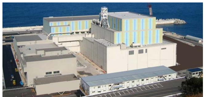
The Chugoku Electric Power Company, Inc.'s Shimane Nuclear Power Station Unit 3, under construction
