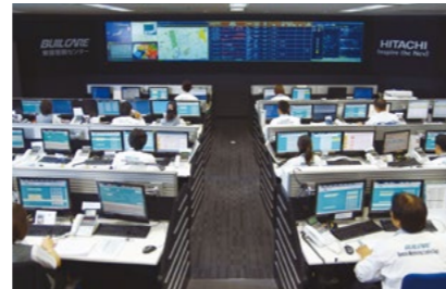
Building equipment is monitored remotely from a call center
